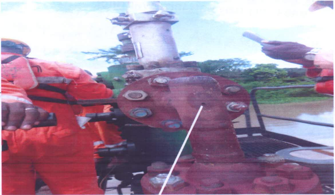
The area were the gas escape through a pin hole leakage at Wellhead Flange Spool, as a result of corrosion.
