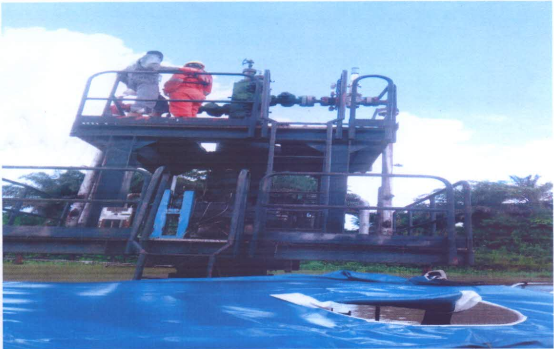
An area view of Obama Wellhead 12 at Obama Flow Station
